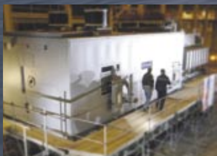
The MT30 gas turbine and alternator package is assembled at the Philadelphia test facility (DD(X) Image courtesy of Raytheon)
