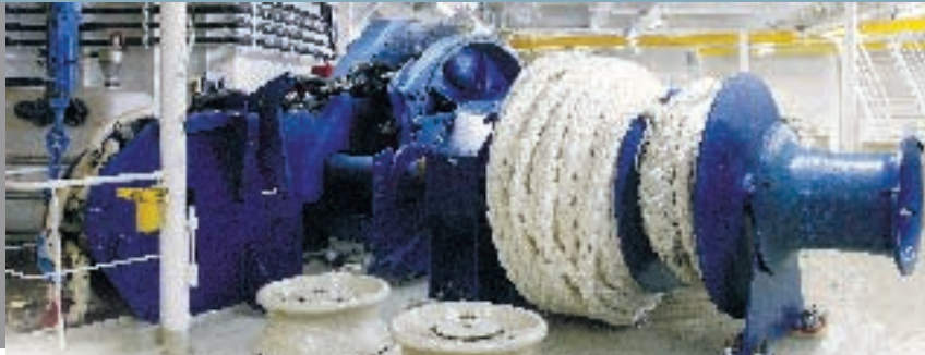
The quietness of electric deck machinery is appreciated on passenger ships
