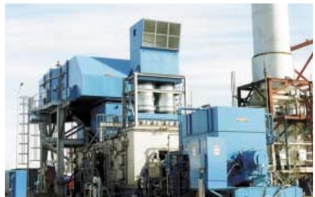
Compact efficient power generation unit
